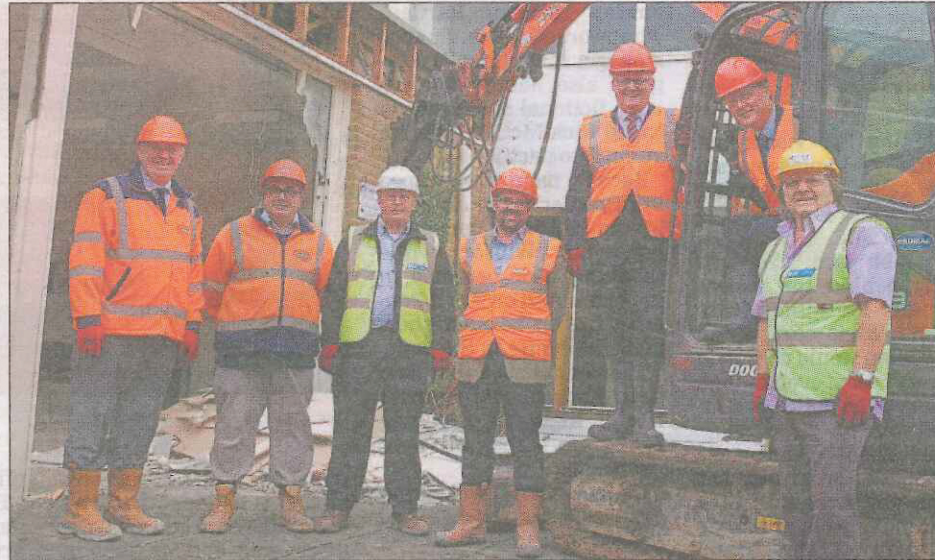
Colin Crowther and Andy Martin, Bouygues UK; Richard Grant, Wessex Demolition, Peter Marsh, Fareham College; Nigel Duncan, Principal; Cllr Seán Woodward; Clint Sexton, Wessex
